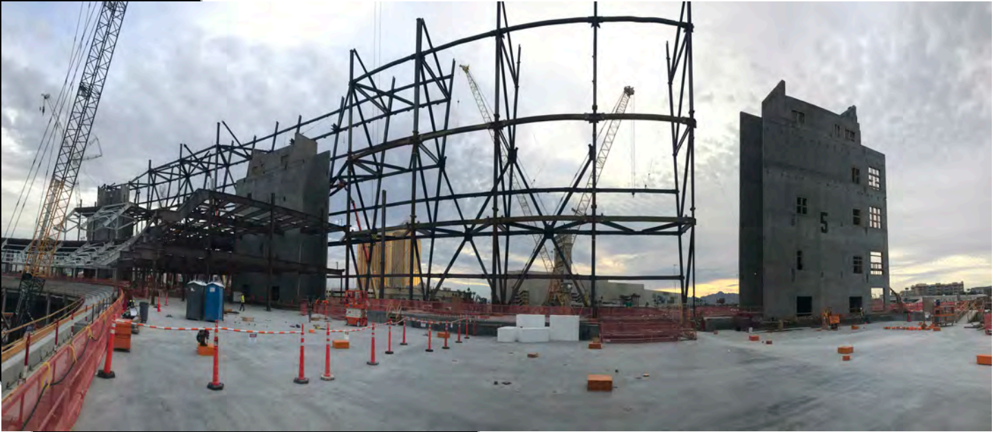
Above: View from Main Concourse, facing East. Below: Metal stud and plumbing rough-in on Lower Mezzanine level.
