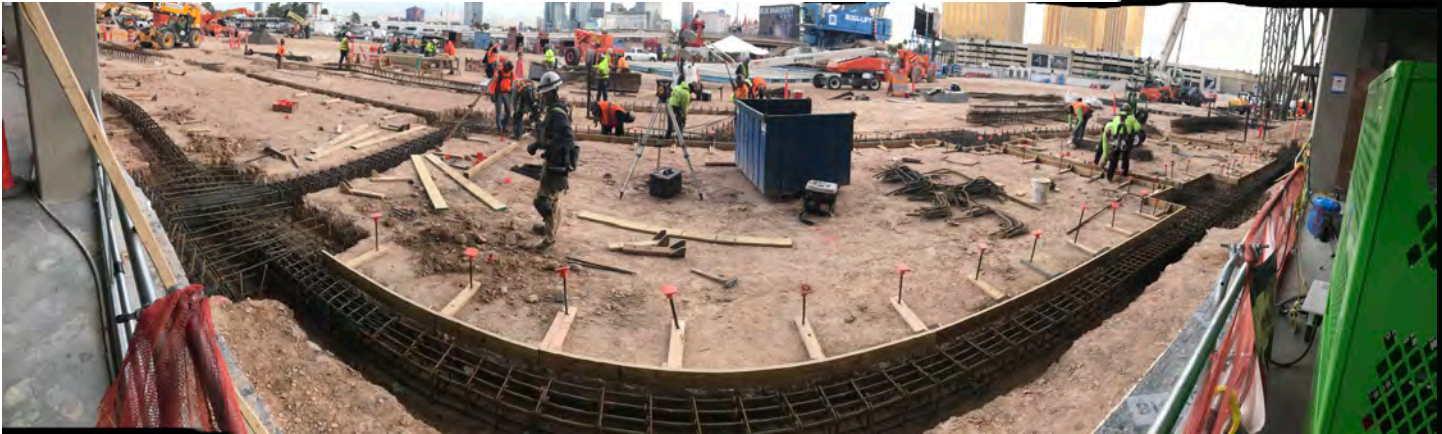
Above: Foundations for North Entrance Grand Staircase. Below: Exterior view of the Northeast corner - vessel steel and man/material hoist tower.
